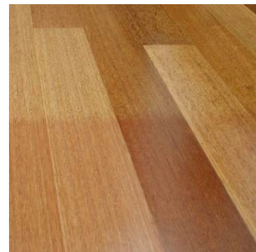
The floor presents as being darker where it had been covered by a rug
