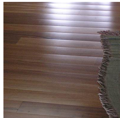
A floated floor crowning in the tropics with a high-density face timber. This degree of crowning is excessive.
