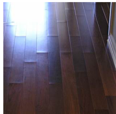
This is an adhesive fixed strand-woven bamboo floor with excessive end-peaking.
