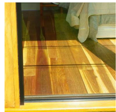
Intense unfiltered sunlight causing checking is an owner responsibility.
