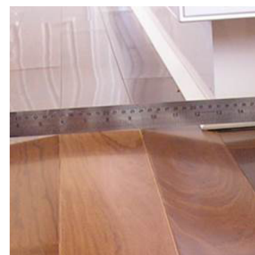
Buckling due to insufficient expansion allowance
