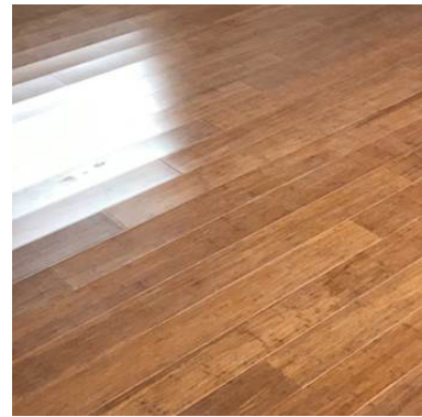
Excessive cupping in a floated bamboo floor from subfloor moisture beneath the floor
