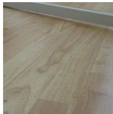
Buckling of the floor inducing creaking and excessive movement under foot.
